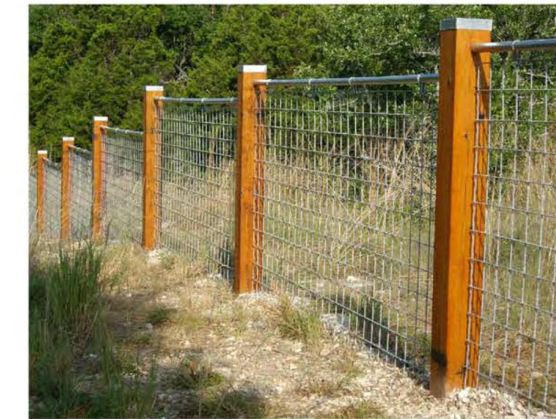
4' Hog wire and wood fencing
